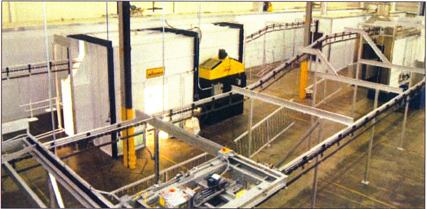
The flexibility of the new coating system is suitable for a job shop environment. Meyer says, "We oversized the line knowing we could fill it up with other work. We needed a good line, so going a little bigger and more capable wasn't a big leap, and it allows us to leverage our investment."
